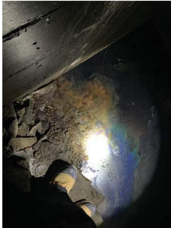
Pictured on the left: hydrocarbons pooling on the floor of the void adjacent to the subsurface concrete water tanks.
