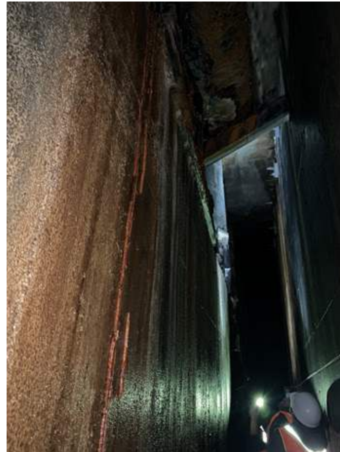
Pictured on the right: The engineering team discovering and examining the remnants of the diesel tank in the void. The tank was for a fire protection pump when the plant was first constructed.
